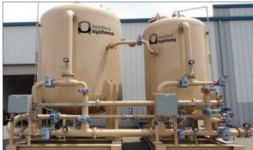
(2) Strong Acid Cation (SAC) Softener Units
