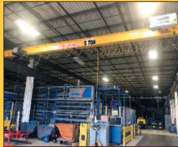
Kone Cranes 5-Ton Overhead Crane
