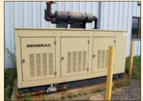
GENERAC BACKUP GENERATOR, NATURAL GAS
