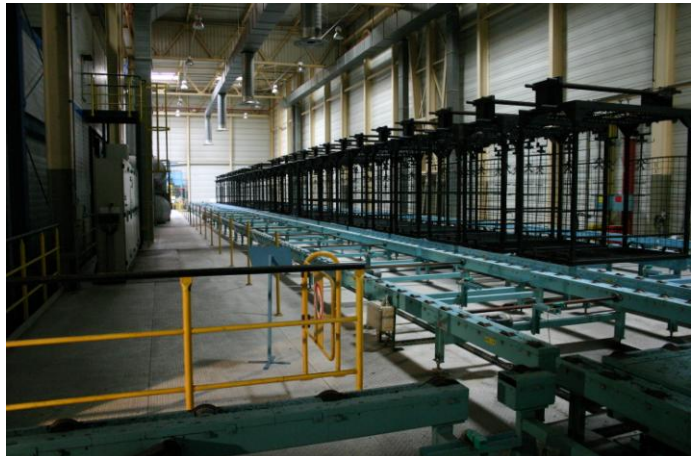
Conveyor System (3 rd Level)
