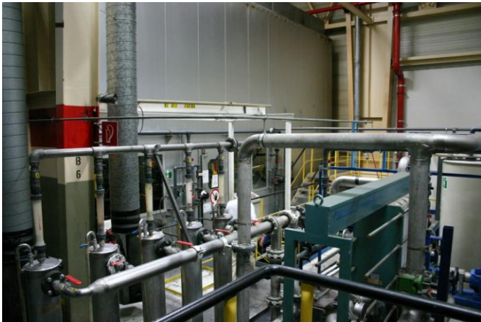
Installation (Paint Unit)
